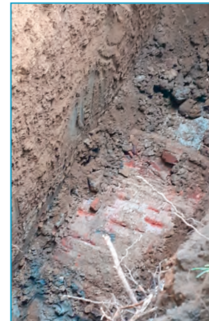
Above: First signs of a man-made structure, apparently the roof of a conduit.
