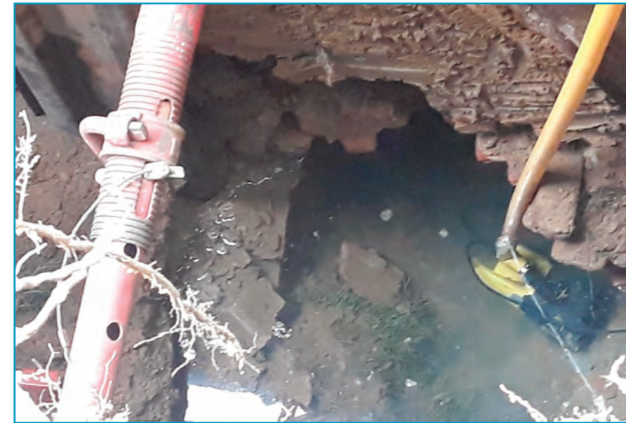
A few more grabs and the brickwork was breached, opening up a void at the bottom of which was running water. Bingo!
